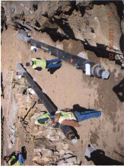
Zone 27 Pump Station Manifold
