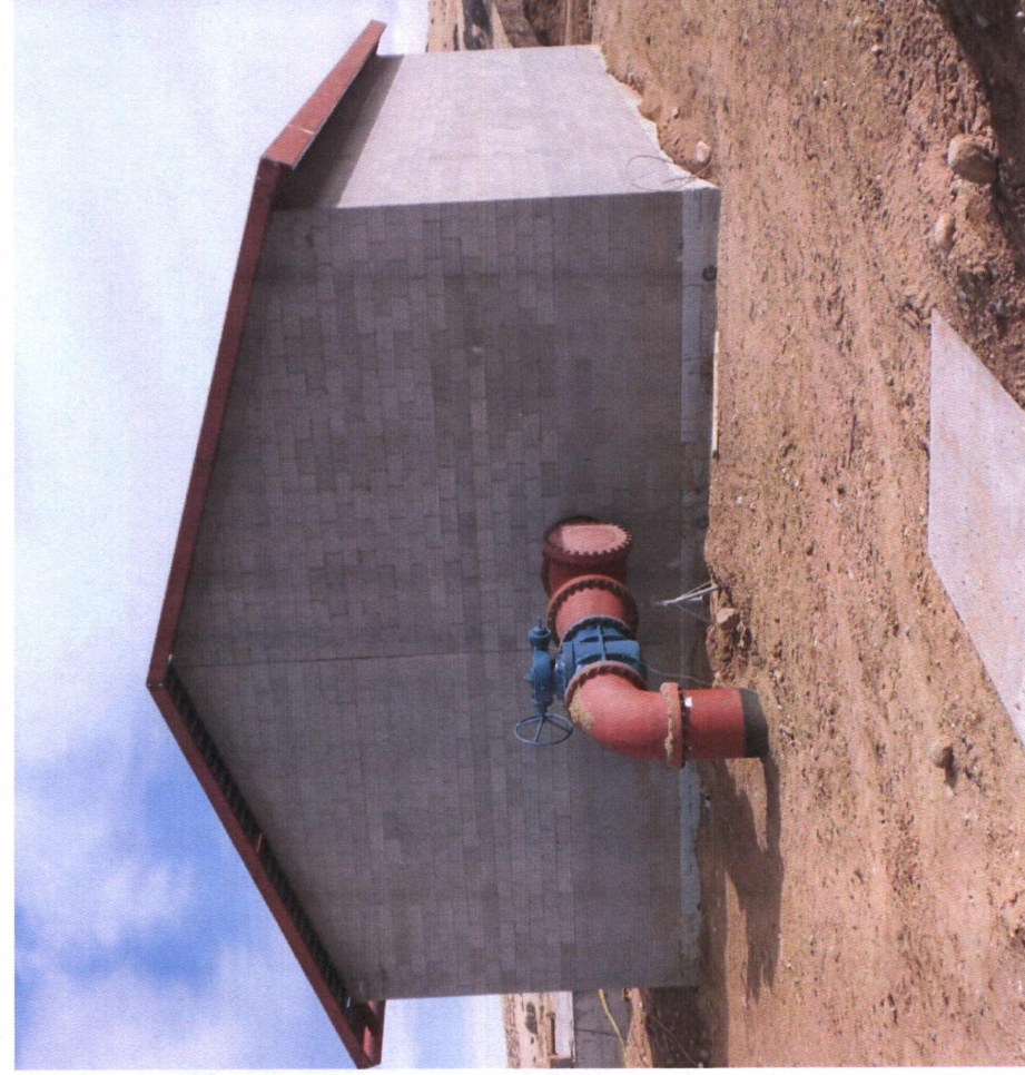
RAS/WAS Pump Station
