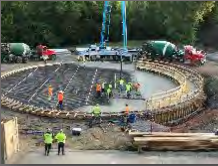
Reading, OH 1.20 MG Sludge Clarifier Metropolitan Sewer District
