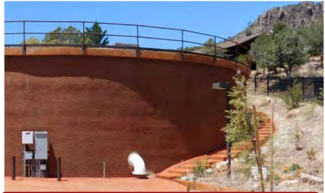
Shown Above: City of Prescott's Zone 27 Tank DN Tanks Project Partner
