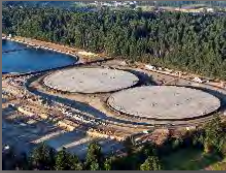
Tacoma, WA 2 – 33.0 MG Reservoir Tanks Tacoma Water
