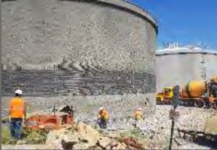
Lawrence, KS 2 – 1.0 MG Water Storage Tanks City of Lawrence Utilities
