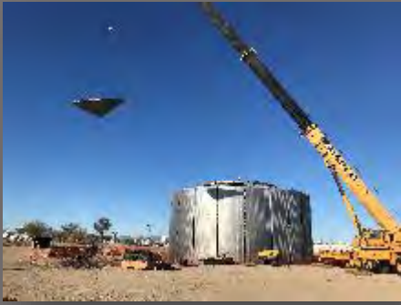
Blythe, CA 1.44 MG TES Tank California Department of Corrections
