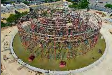
San Antonio (Bitters), TX 5.0 MG Water Storage Tank San Antonio Water Systems (SAWS)
