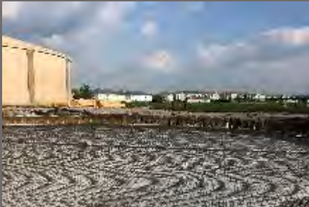
Crown Point, IN 3.0 Water Storage Tank City of Crown Point
