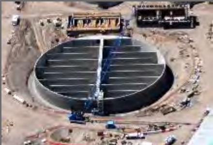
Tucson, AZ 8.9 MG SBR Tank Pima County Wastewater
