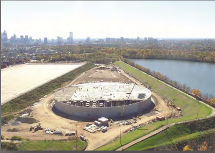
Philadelphia, PA 3 – 32.0 MG Water Storage Tanks Philadelphia Water Department
