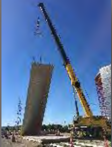
Garland, TX 6.0 MG Water Storage Tank No. TX Municipal Water District (NTMWD)
