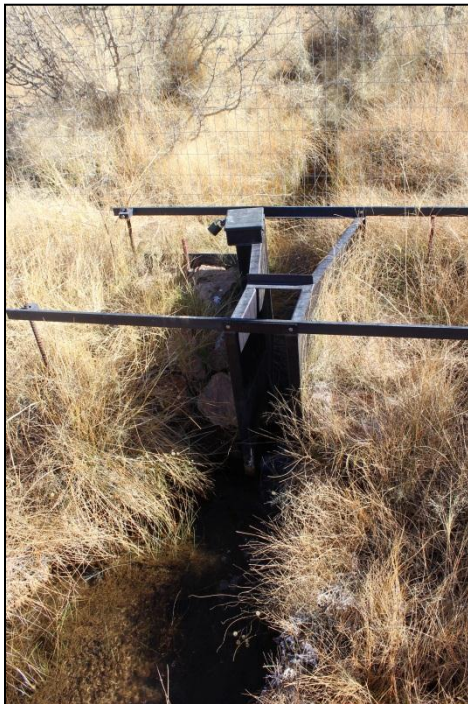
Figure 19 Another view of the flume used to monitor low flows at a site. Photo taken ~1.5 years after installation. Photo Credit: SRP, November 2012.
