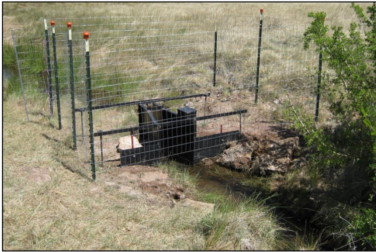
Figure 18 Example of a small flume used to monitor low flows at a site. Photo taken shortly after installation. Photo Credit: SRP, June 2011.
