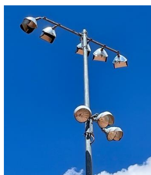
Old, inefficient sports field lighting with poor light quality
