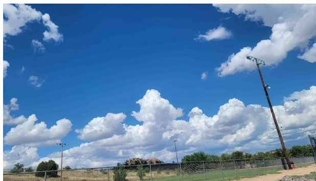
Figure 5. Heritage Park Baseball Field LED stadium lighting offers multiple advantages of extreme power savings, impact resistance, long service life, low maintenance requirements and excellent light uniformity and quality.
