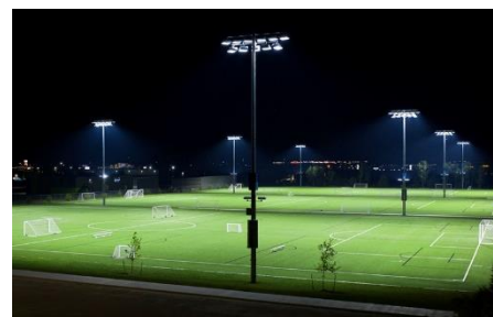
Modernized LED Sports Field Lighting
