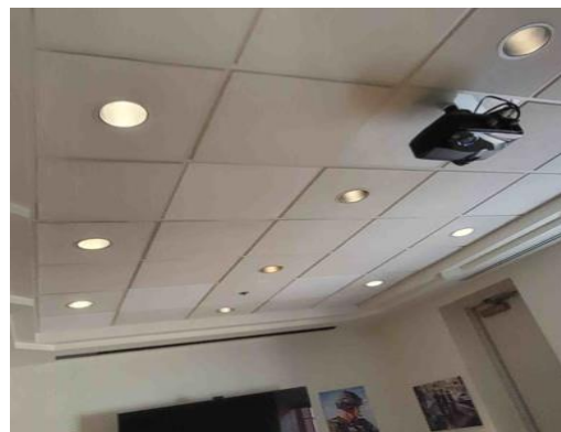
Figure 1. CFLs at Police Dept LED bulbs are a cost effective solution to improving light quality within conference rooms and other spaces
