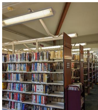
Inefficient Lighting Systems
