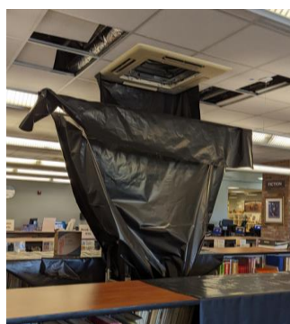
HVAC at the end of useful life
