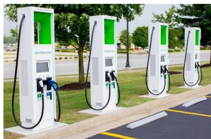
EV Charging Stations
