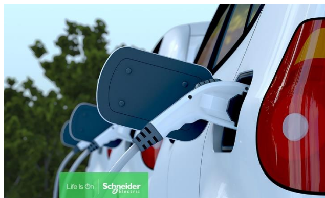
Figure 12: Electrical Charging Infrastructure. EV charging stations maximize convenience for EV drivers and station owners.
