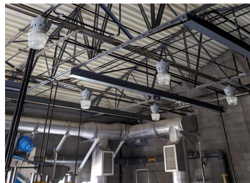
Figure 2. HPS High Bays at Airport WWTP LED fixtures would provide energy savings as well as reduced maintenance hours
