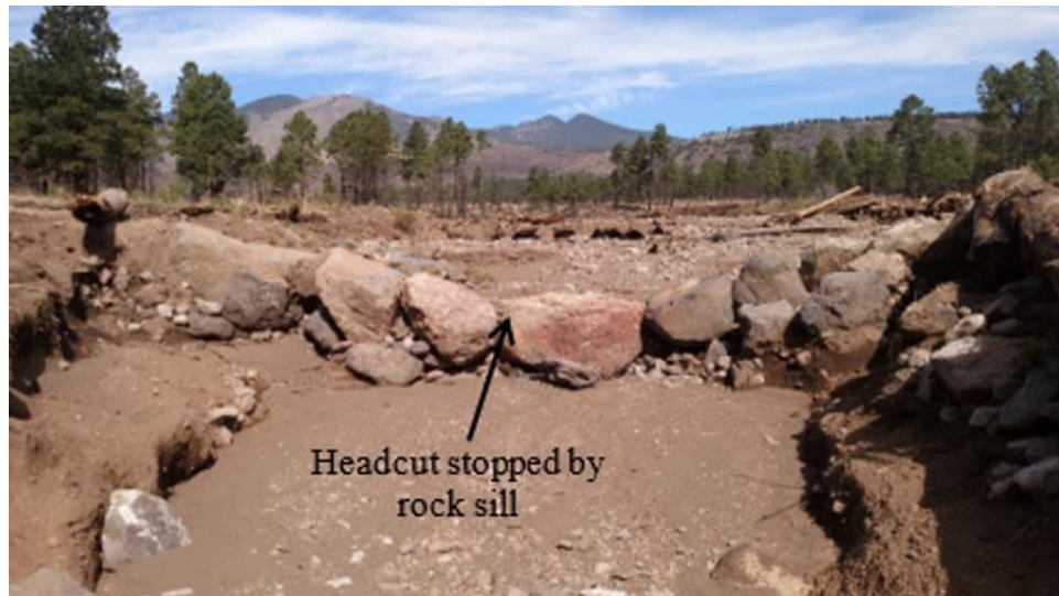
Figure 41. A rock sill maintains the upstream channel gradient in a post-fire burn area. This rock sill remained intact following a 1000-year storm event on the upstream watershed.
