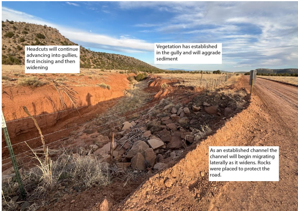
Figure 15 A headcut coming from Williamson Valley Wash and endangering the road
