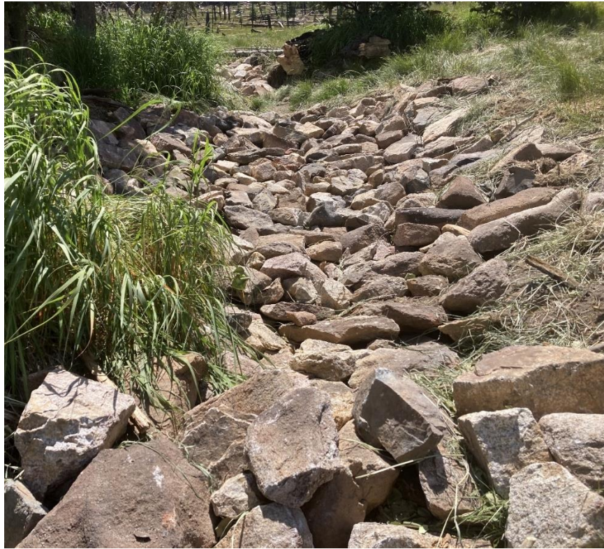
Figure 46 A rock rundown constructed with a brush mat underlay. NOTE: Surface water can flow into this structure because the middle of the structure is at/or below grade. Also, note how the sides of the structure follow the channel up the slope- failure to do this will enable surface water flows to bypass the structure.
