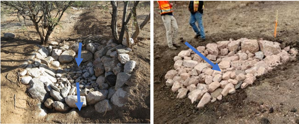
Figure 44. Zuni bowls installed at headcuts with blue arrows indicating the direction of flow.
