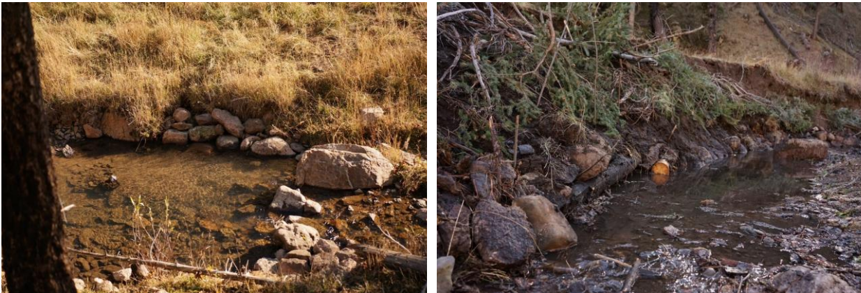
Figure 40. Bank armoring. Left: bank armoring only was used to fill small sections of unstable banks in an otherwise stable channel. Right: bank instability on the cut bank was armored and one-rock dams (not seen) were installed above and below to promote channel stability while toe rock prevents further bank erosion. Note the use of logs in conjunction with rocks.
