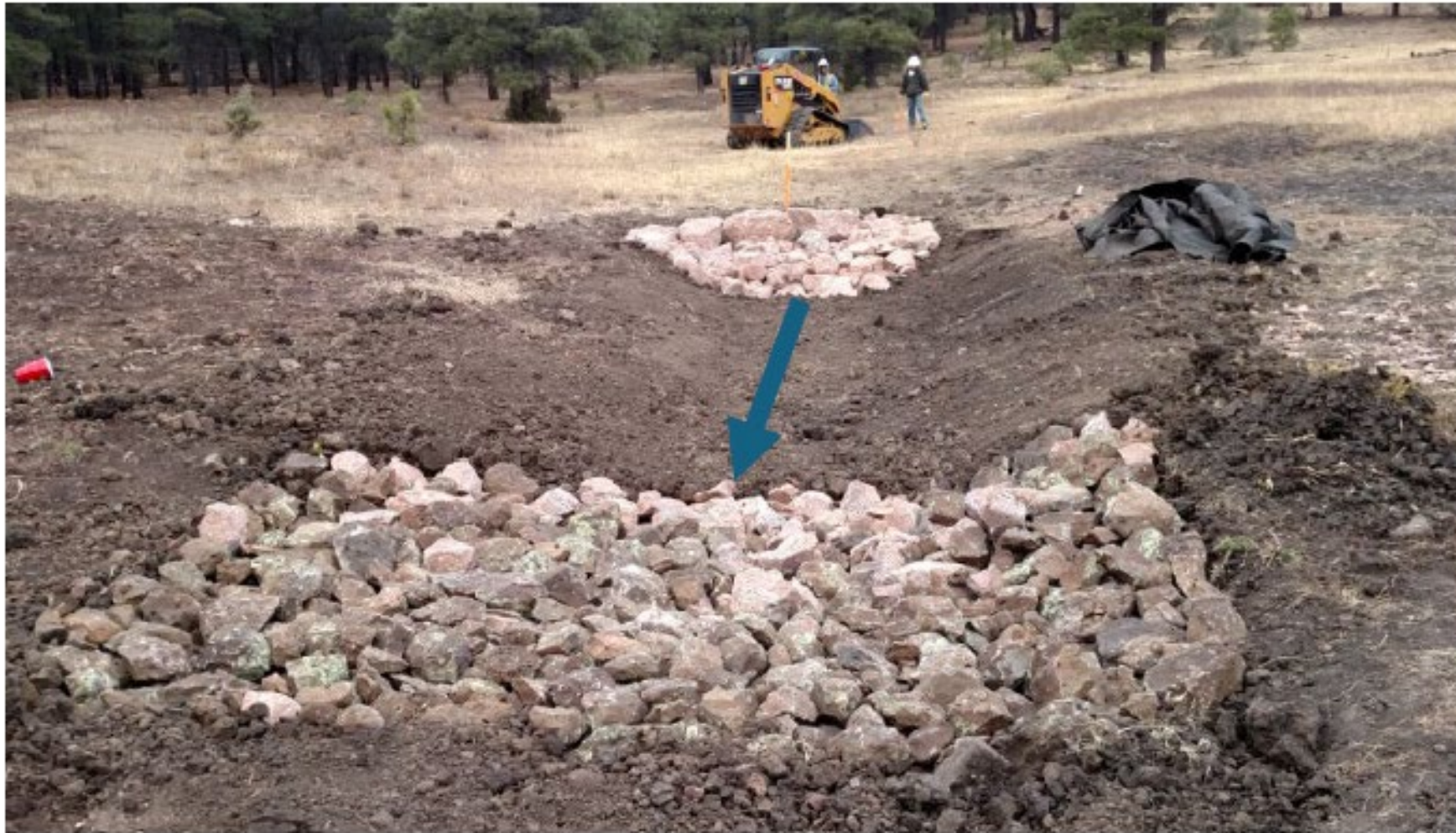
Figure 6. Example of a Zumi Bowl and one-rock dam built in series to arrest a headcut and begin channel aggradation. Arrow indicates direction of flow.
