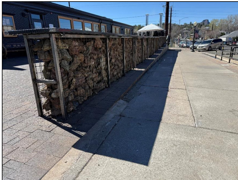
Figure 2. Image of gabion wall currently constructed at 202 South Montezuma Street, facing west (City of Prescott 2026).
